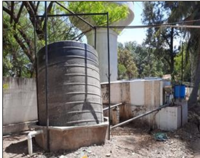
Solid waste utilization in Biogas Plant.
